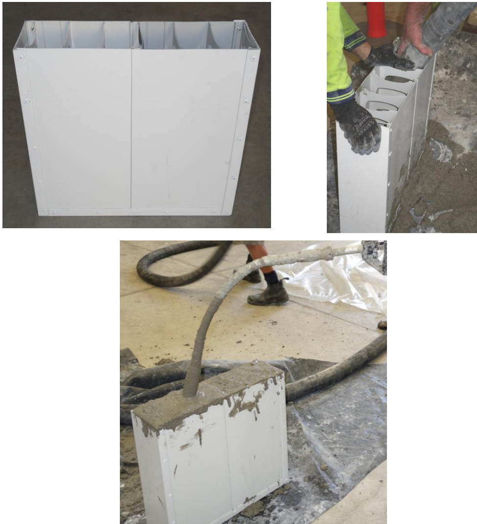
Figure 3 Preparation of Rediwall block section of the wall panel for water permeability testing
